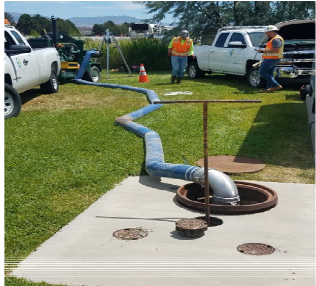
Figure 16: Pump by-passing the station from the inlet manhole to the pressure manhole.
