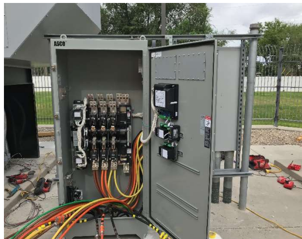
Figure 8: New Automatic Transfer Switch Panel
