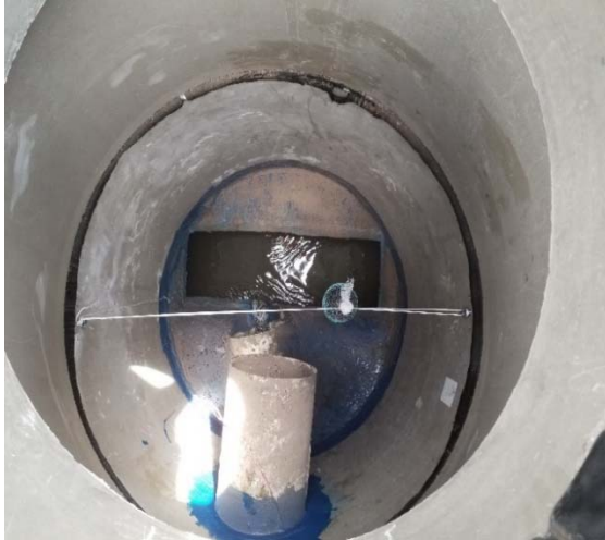
Figure 12: Depicts the H 2 Sorb suspended in a manhole
