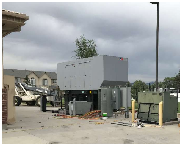
Figure 7: New Well 16 Generator
