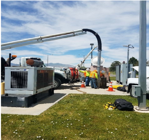
Figure 15: Using the Vactor truck to vacuum the grit and debris from the bottom of the wet well.
