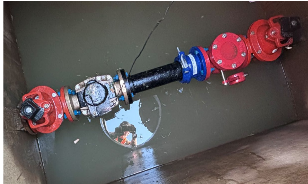
*Before and After pictures of the Large 3" Meter at the Pioneer Medical Building replaced after hours to accommodate for continuous care.
