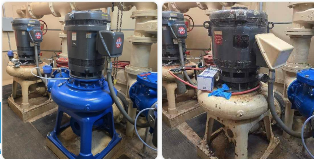
New vs. Old pump at East Rec
