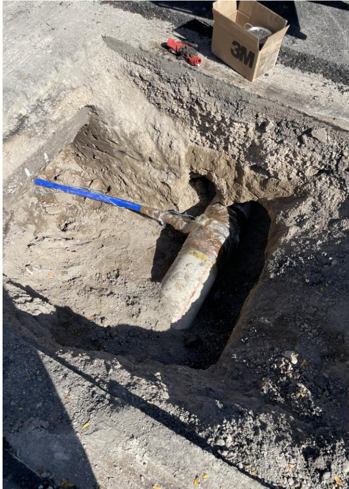
2" water lateral connection on 12" main
